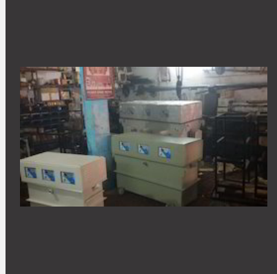
Oil Cooled Servo Stabilizer 75 KVA
